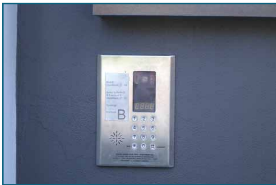
Entry phones restrict and control access to residential complexes.
